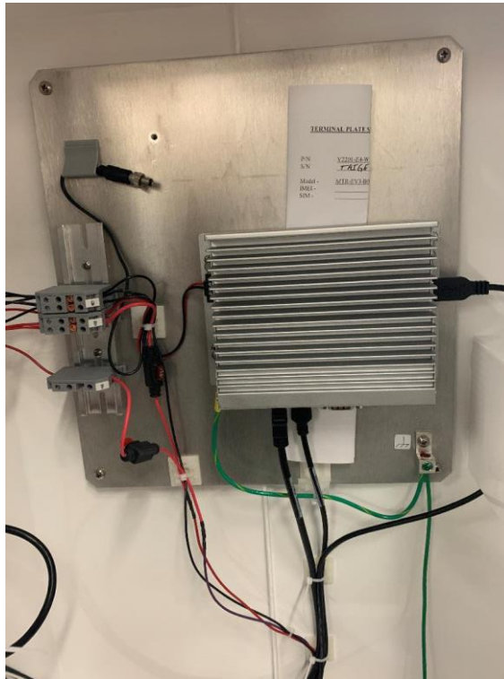
Upper M4000 Component Wiring
