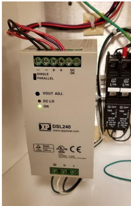
Figure 10 - Power Supply Mounted and Wired
